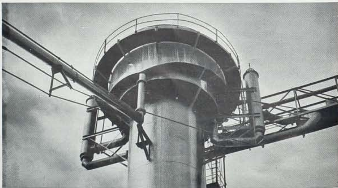
Tower of large light oil scrubber installed at East Station during 1937. It operates in parallel with the original scrubber there.
