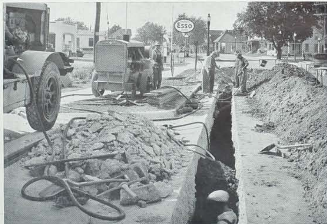
Typical gas distribution construction job, East Avenue near Winton Road. Replacing 6-inch medium pressure gas distribution line with 12-inch line to provide greater capacity in the East Avenue district. Modern equipment aids greatly in speeding such work and cutting to a minimum the time necessary to accomplish necessary construction work.
