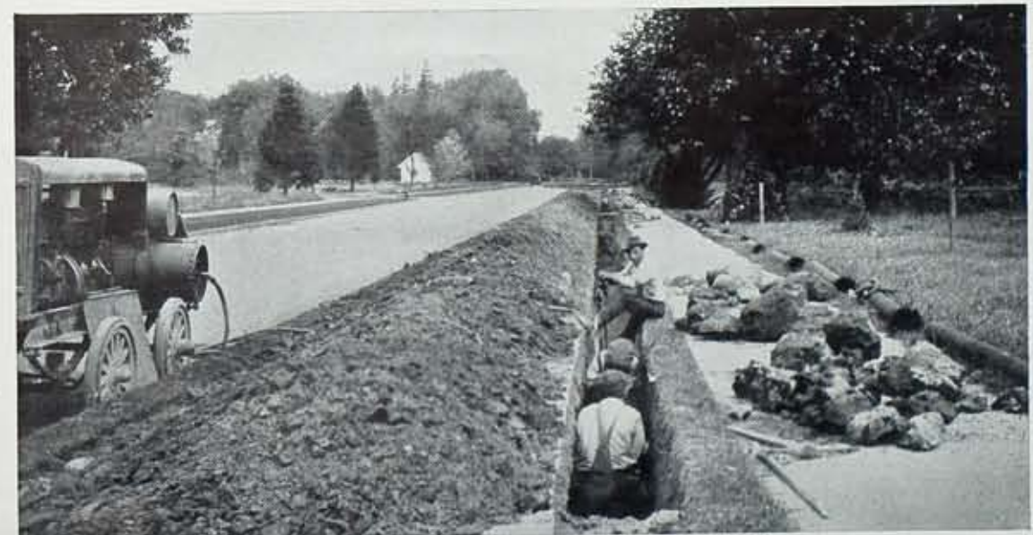
Installing gas mains along one of Rochester's newer residential streets. The Gas Street Department makes every effort to prevent any damage to property. Canvas is laid over lawns to keep the piled-up soil from harming it, and after the mains are laid the sod is carefully replaced in its original position.
