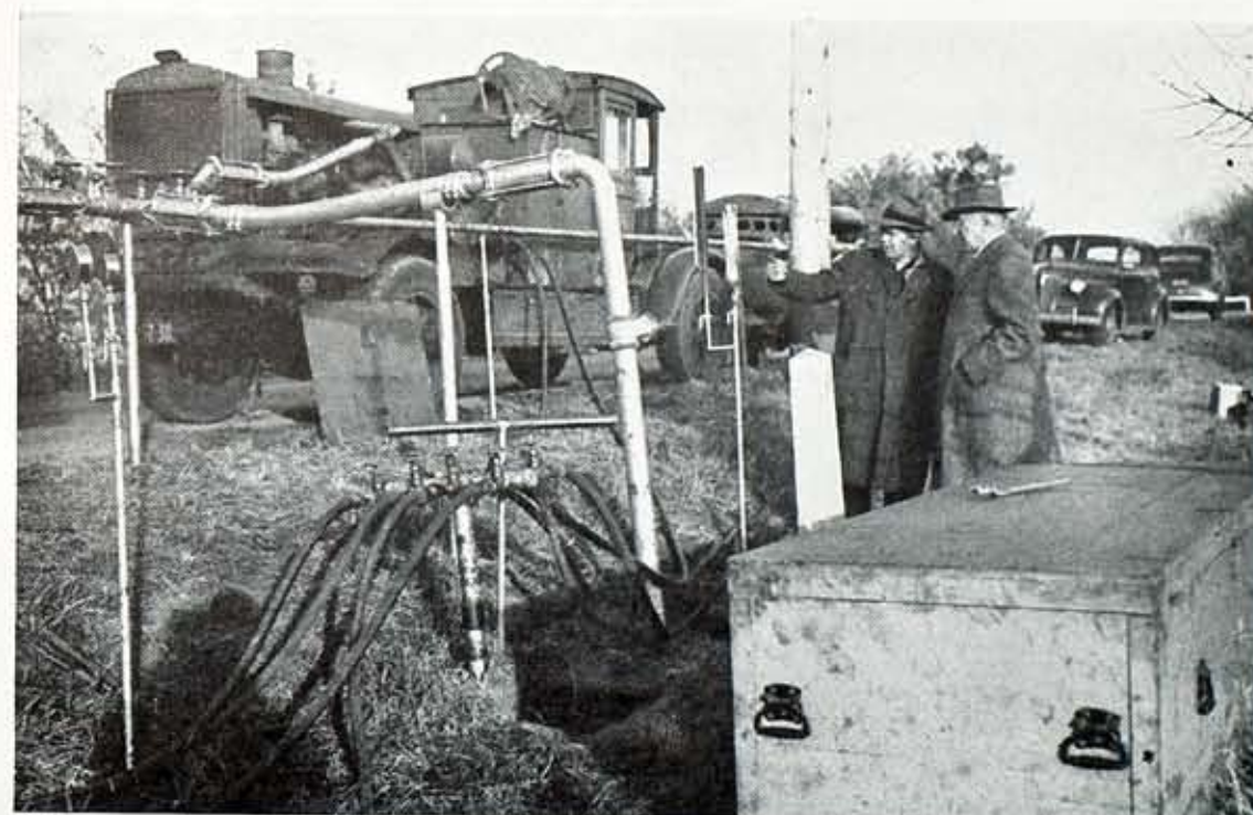
Don MacCollum, left, pointing out features of the Ridge Road gas pumping installation to Dick Hoddick, Superintendent of Gas Distribution.
