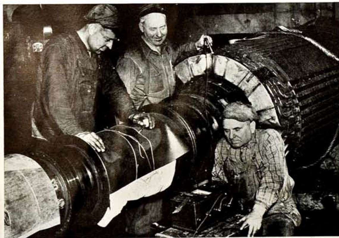
Shown left to right are Harry Sheetz, George Robinson, and Everett Ferge. They are checking the coils on No. 7 Steam Turbine at Station 3 for grounds. They are using an apparatus known as a meggar, which goes after a "short" like a ferret after a rabbit.
