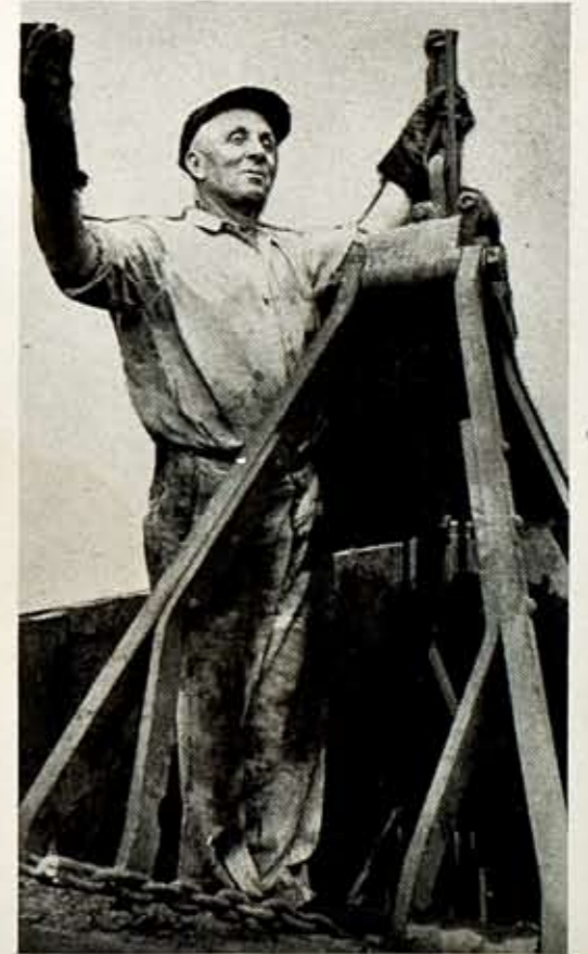
Bruce McCahan, General Maintenance, gives the crane operator the high sign and another shovelfull of dirt is subtracted from a new excavation.
