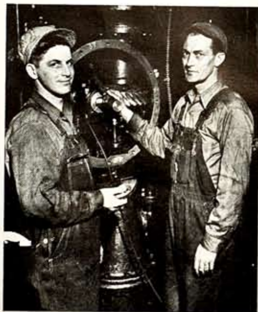
Teddy Cornelio and John Cross, left, are seen installing new worm gears, part of equipment made use of to modernize the governor drive on the 15,000-KW turbine at Station 3.
