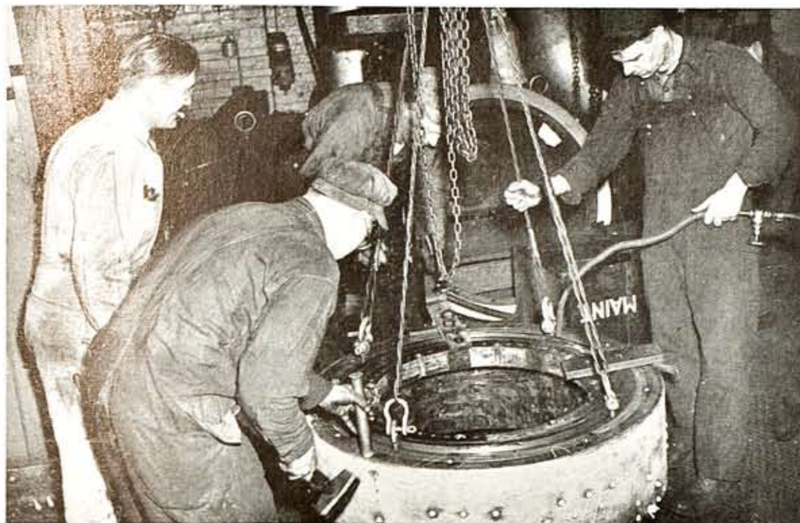
Shrinking a turbine generator ring onto the field is a precise operation requiring expert handling. In picture are shown, left to right, Carl Wicks, of the General Electric Company, Everett Ferge, Wally Bond, and John Allen.
