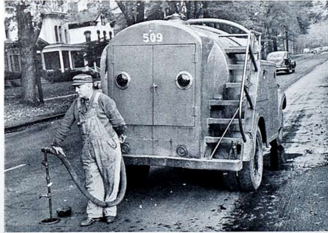
James Failing pumping out a gas "drip" on his morning route along Lake Avenue. The truck's engine does the pumping. Note the large round signal lights which flash a red warning while truck is in operation on a busy thoroughfare.
