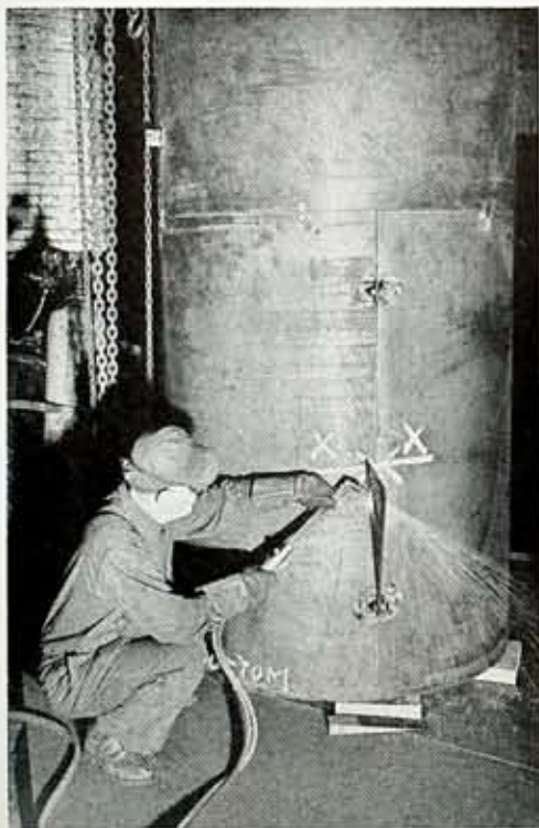
Henry DeRoller, expert Company welder beginning to cut up this large steel tank into geometrical sections in order to get it into Station 11, where it was reassembled and rewelded.
