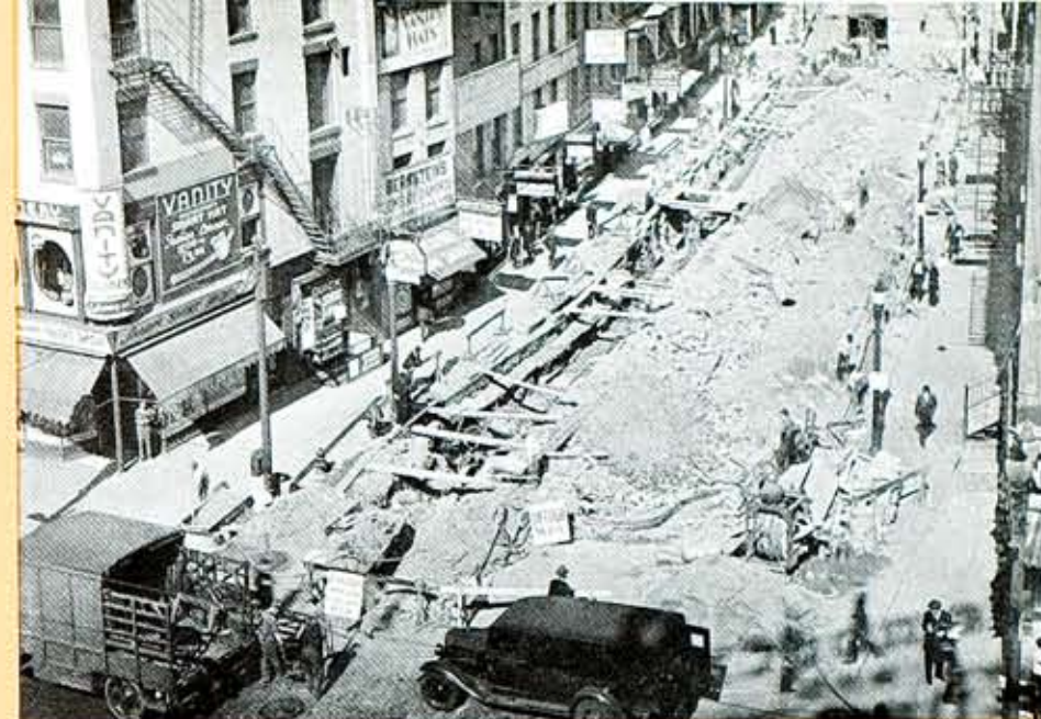
Reconstruction of gas mains in connection with the paving of Front Street gave the gas street Department a real job.
