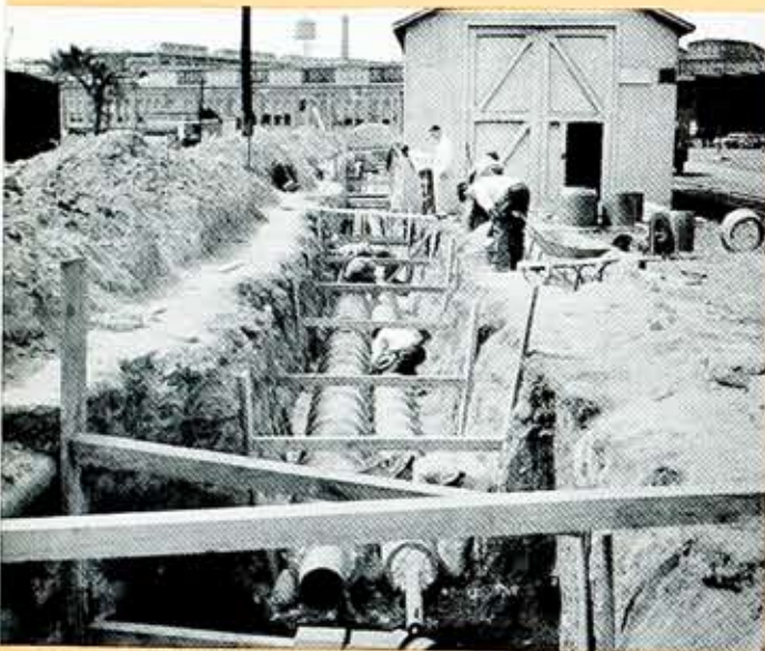
Laying the steam line to the plant of the Pfaunder Company, Lincoln Park.
