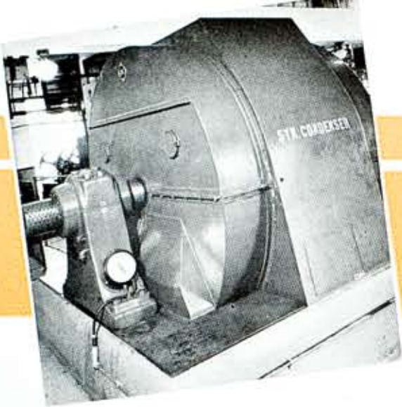
5,000-Kva synchronous condenser installed at Station 1 on the 4,150-volt bus.
