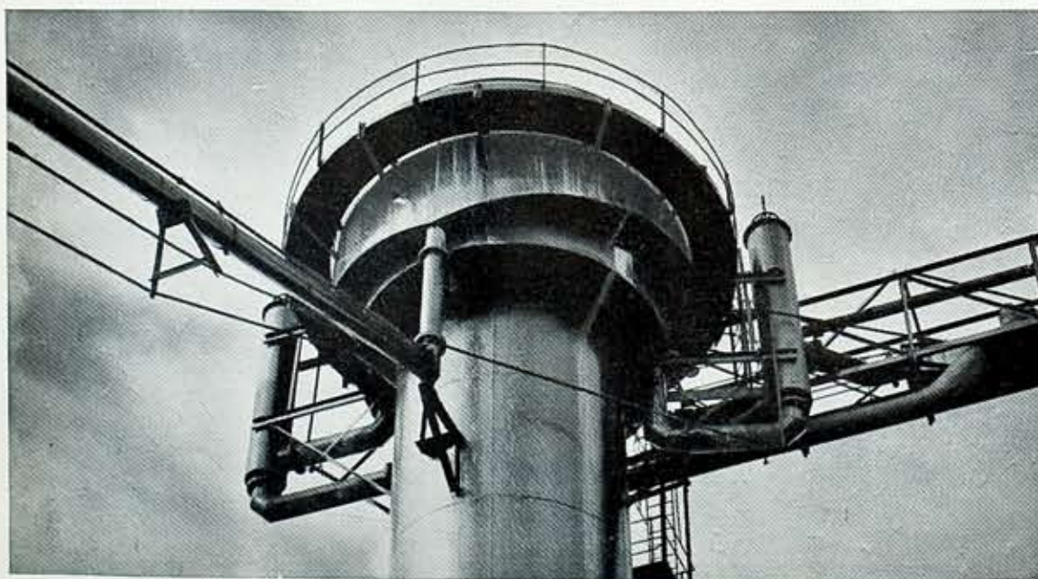
Another view of the Thionizer tower, showing pipe through which the released sulphur is transported to the building nearby where it is put through a filter press.
