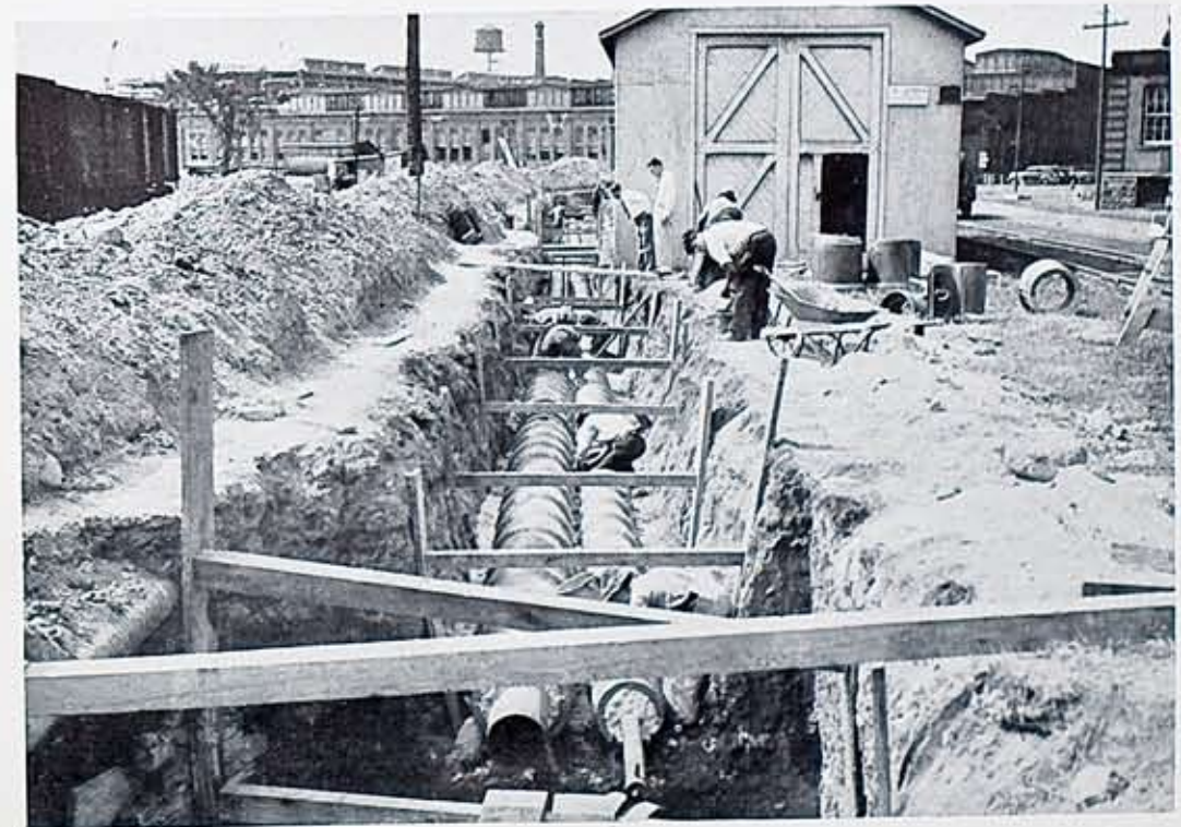
Approaching the existing buildings of the Pfaunder Company the 12" low-pressure and 4" high-pressure steam mains are shown encased in Ric-wil tile conduit with Rockwool insulation.
