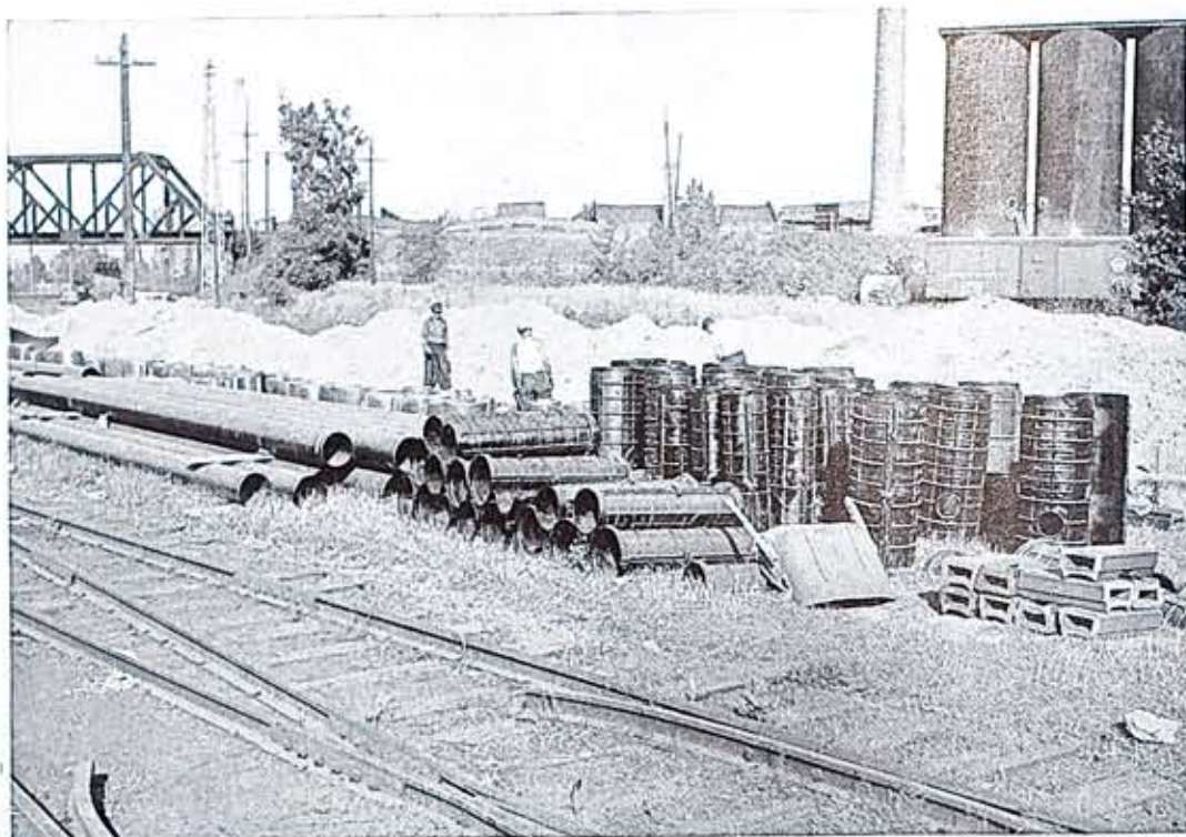
Some of the materials which go into a steam main. Part of the heavy 12-inch steam main and cast iron Ric-wil conduit used beneath the seven branch railroad sidings along the route.
