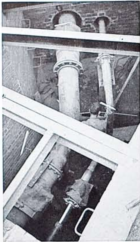
View into one of the steam manholes showing expansion joints provided on the steam mains and anchor points at change of direction in the line. Drip points are also provided to remove from the steam any moisture which may have accumulated so as to insure the delivery of clean, dry steam to the user.
