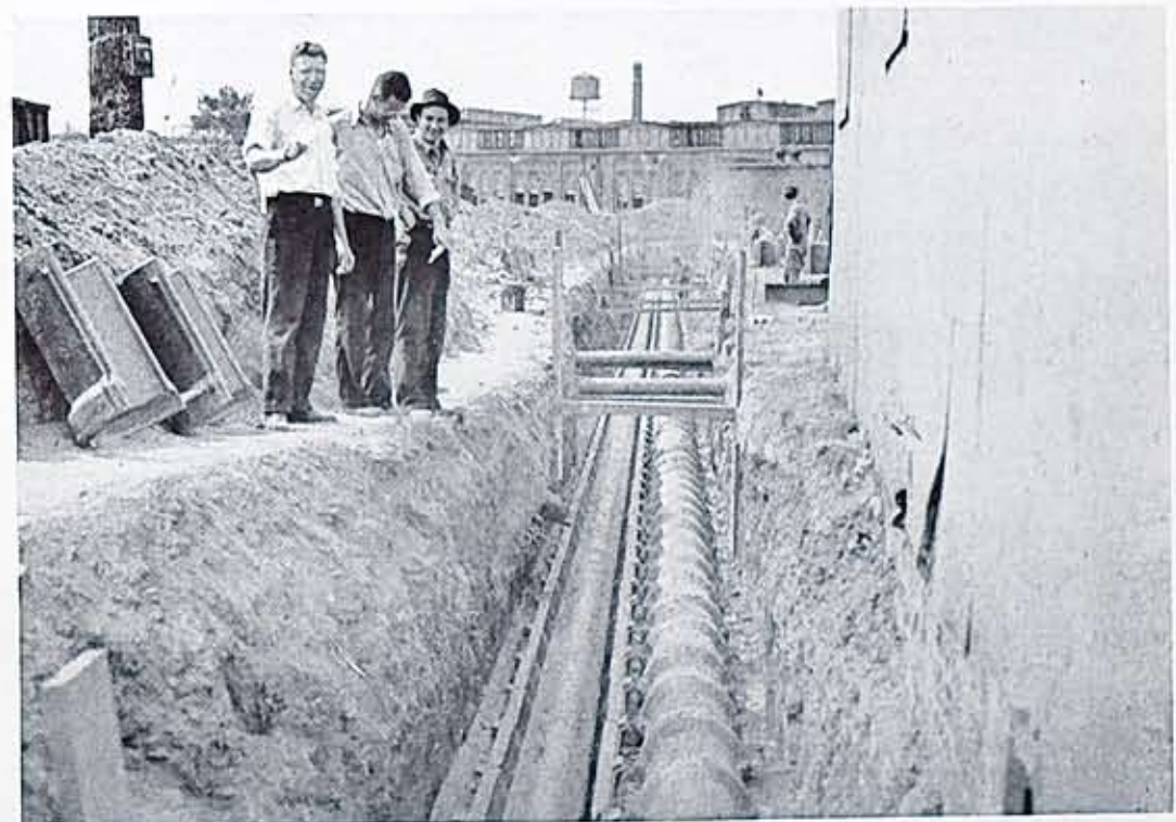
The mains were installed under the personal supervision of Sam Springer of the Steam Distribution Dept. in charge of Julius Schenk and Emery Powell and under the personal supervision of Don LePine of C. P. Ward, Inc., who are shown inspecting their handiwork.
