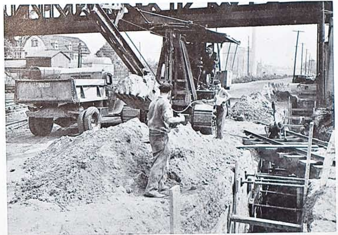
C. P. Ward's trench diggers at work on excavation at commencement of steam mains near northwest corner of General Railway Signal Company's property. From this point the existing steam mains extend along the main line of the New York Central Railroad to the Company's Lincoln Park Plant which is seen just beneath the B. & O. Railroad Crossing.
