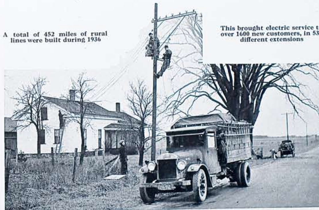
A total of 452 miles of rural electric lines were built last year. This shows a typical scene, with contractor's men stringing wires, trimming trees and installing the service from pole to farm home.
