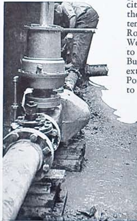
Duplicate, pressure controlling regulator, installed at East Avenue and City Line to insure quality gas service beyond the City Line and to some streets off East Avenue.
