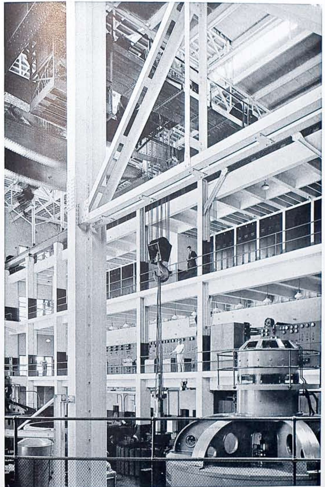
Section of Interior of Station 5 Hydraulic Plant, Lower Falls of the Genesee River.
