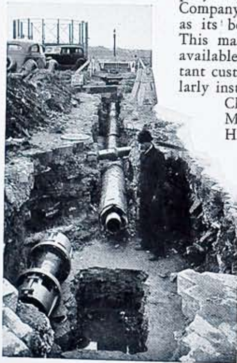
Section of 10-inch high pressure steam main through Bartholomay Brewing property and extending to Station 34, showing excavation for manhole which will contain double expansion joints, shown at left.
