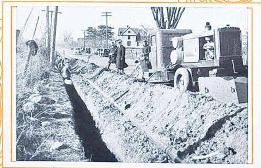
Scenes along the new Chili Avenue gas line extension. Top: Tough going through a rock fill, showing gas pipe ready to be dropped into trench. Center: When the line took to the field it was easy going for the big digger. Bottom: Where the line approached the West Shore Railroad crossing. A stretch of hand digging along the main highway.
