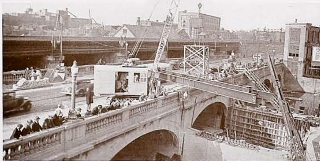
Transferring the superstructure from a truck to its position at the dam site. The New York Central railroad bridge is seen in the distance.
