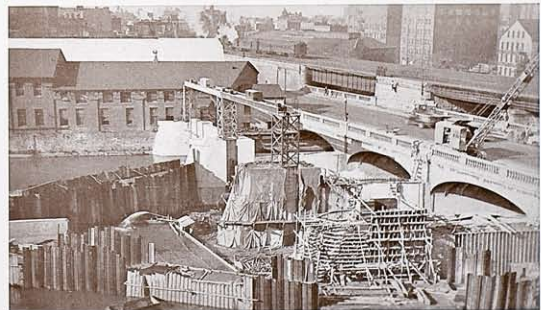
Cofferdam and concrete forms for gates two and three. Gate number one at extreme left in the picture is seen in its completed form.
