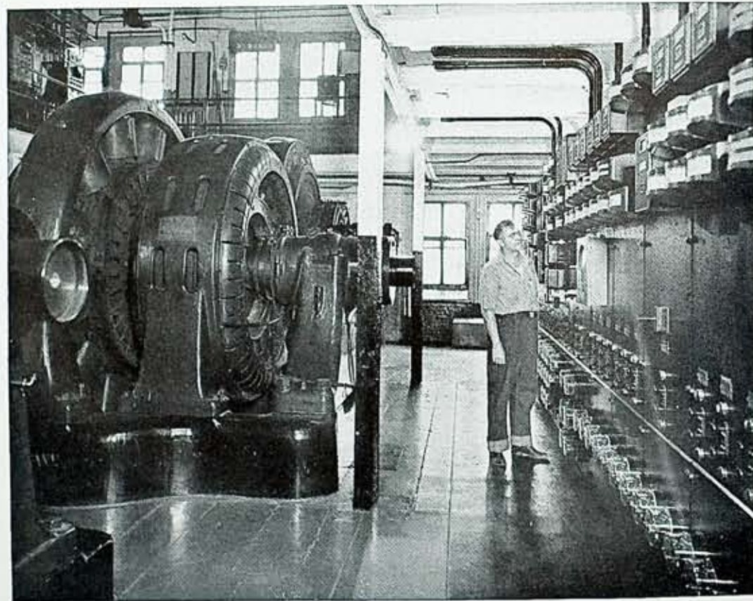
One word describes the plant cleanliness at Station 35. It is—immaculate. Everything is shiny-clean, even the tops of the generators and the corners and crannies. The West Point white glove test would have no terrors for a plant like this.
