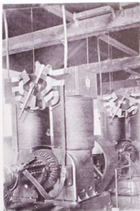
This Edison Bi-polar generator was thought to be "big stuff" in 1890 when it was termed a "Jumbo" unit. It weighed about 17 tons and generated about 10-kw. of electricity per ton, approximately. Present day generators, such as shown in illustration on page 263, generate approximately 250 kw. per ton because of the refinements in the electrical art and greater all around efficiencies.
