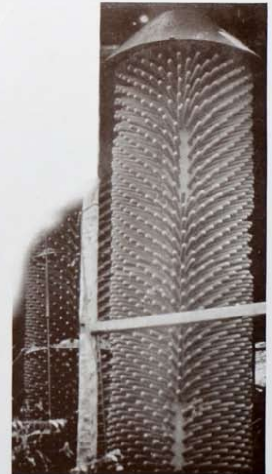
Until 1902 eleven boilers of this "porcupine" type were functioning at old Station Two. They were of 125-pound pressure and evaporated 10,000 pounds of steam per hour. These boilers were prone to foam, carrying water over with steam to reciprocating engines, sometimes knocking out a cylinder head. The circular furnace was hand fired through three doors. Water tubes were great scale collectors. Potato skins and "quack" boiler compounds were the inefficient antidotes for this trouble.
