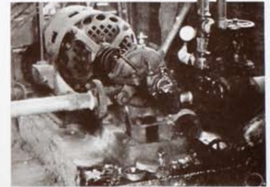
Electrically operated centrifugal pump on Van Lara farm, Farmington, which serves ten acres of irrigation.
