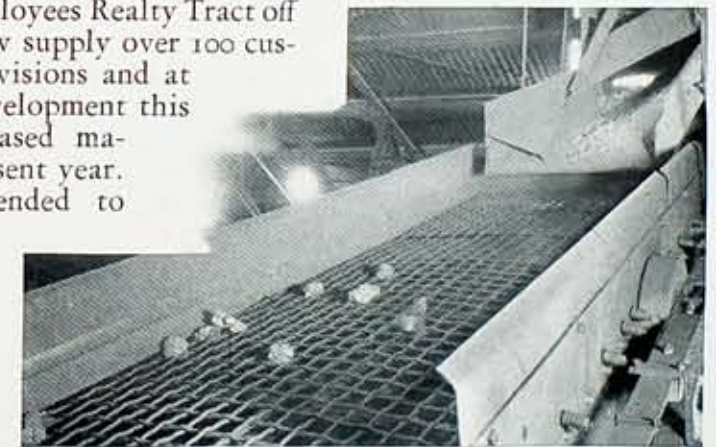
Section of electrical coke screening equipment at the Coke Bins, where screening, sizing and other operations insure coke of uniform quality.
