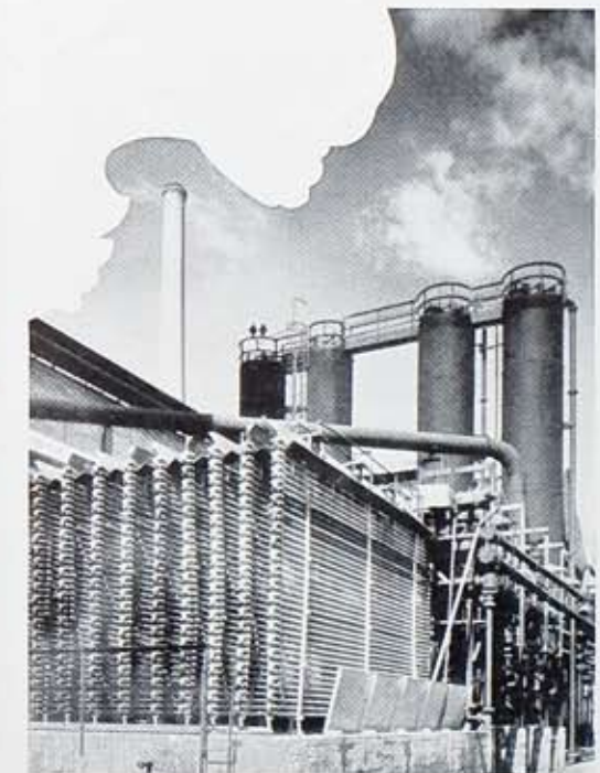
Cooling coils at coal gas condensing plant, West Station, containing four miles of pipe.
