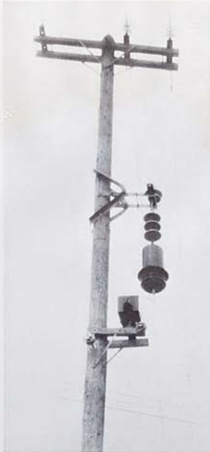
Coupling capacitor and spark gap located at Canandaigua, N. Y.
