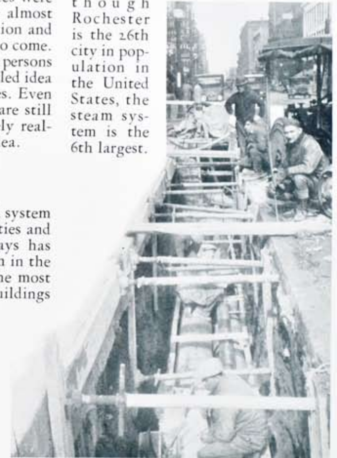
Progress of underground steam construction. Electric welding crew has completed installation which consists of three pipes at this location: a 14-inch low pressure steam main; an 8-inch high pressure steam main and a 6-inch pipe through which the condensed steam is returned to the station. Insulation crew is at work in preparation for the final construction of concrete box forms, back fill and re-paving.
