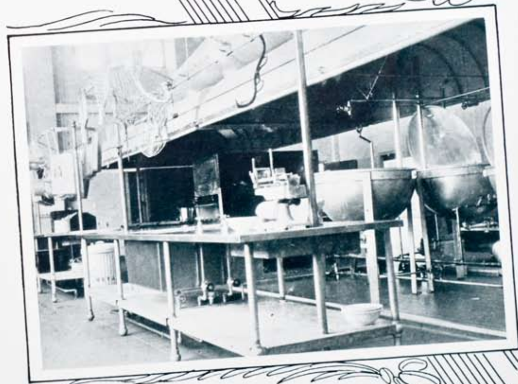
Top, view of bakery with its modern electrical equipment such as mixers, proof box, electric range, kettles, freezing cabinet, ice machines and freezers. This bakery is capable of taking care of the requirements of a total of 468 patients.
