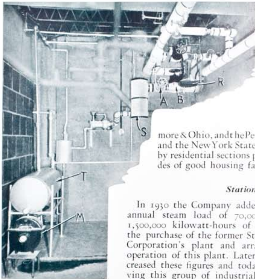
Typical Steam Service and condensation meter installation showing simplicity of complete apparatus which eliminates necessity for boilers, coal storage, chimney, etc. The Company's steam service enters the building through the wall back of the separator (S) which insures high quality steam in the customers system. Steam flows through the Company's service valve (A) and the customers service valve (B) to the customer's regulating valve (R) which controls the pressure on the customer's heating system. Returns from the radiation in the form of condensed steam are collected in the receiving tank (T) and measured by the direct reading condensate meter (M) which gives a continuous record of heat use.
