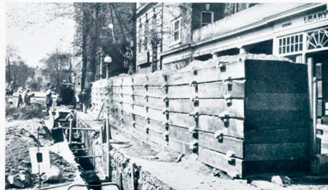
Steam construction in progress in Chestnut Street. This view shows the method used in caring for the dirt removed from the trench, and to avoid interference with pedestrian and vehicular traffic and in the interest of safety. This dirt is used later for back-filling the trench.
