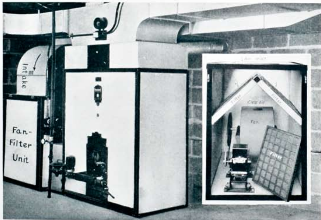
Gas heating installation in a Rochester home. At left of heating unit is the fan-filtering unit, which is shown with case off at the right. Any home can easily use existing air circulating facilities to filter and cleanse the home's air supply and help keep it cooler in hot weather.
