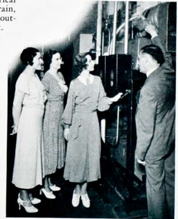
Mr. Lundgaard explaining the operation of the Carrier refrigerating unit in the basement of the Gas and Electric Building to, left to right, Miss Veronica Leonard, Miss Kendelen and Miss Dorothy Maslyn. This unit supplies cooling equivalent to melting 50 tons of ice every 24 hours.
