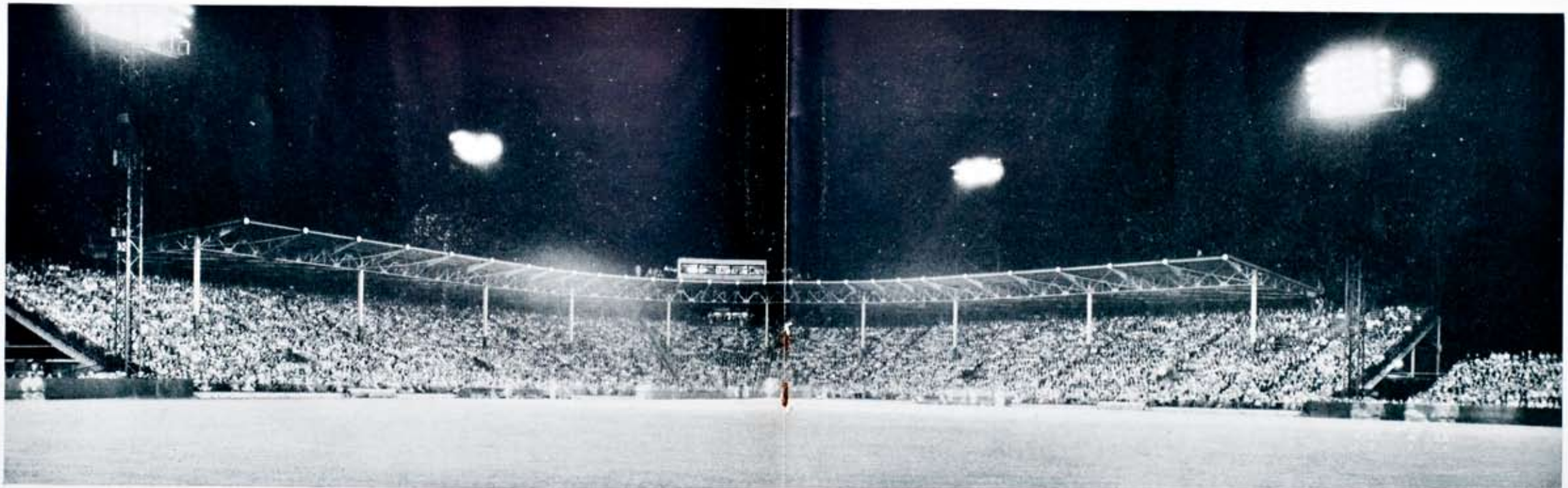
Scene at one of Rochester's first night baseball games under the new lights, last season, when more than 16,000 persons were in attendance. This lighting job was installed by the Dwyer Electric Company, of Rochester.
