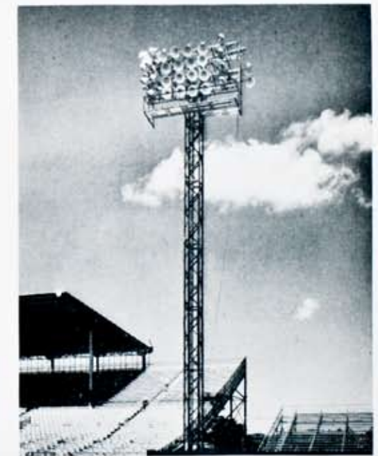
Right: Hundred-foot outfield tower having both open and closed type of lamps, the former having 2 1500-watt lamps each, and the latter, one 1000-watt lamp each.
