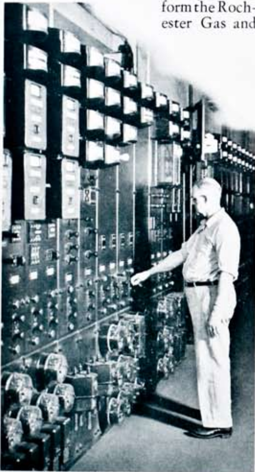
When the operator shown above pulls out the small knob on a switch, over 400 electric street lamps, or about a mile of lights, are simultaneously put into service.
