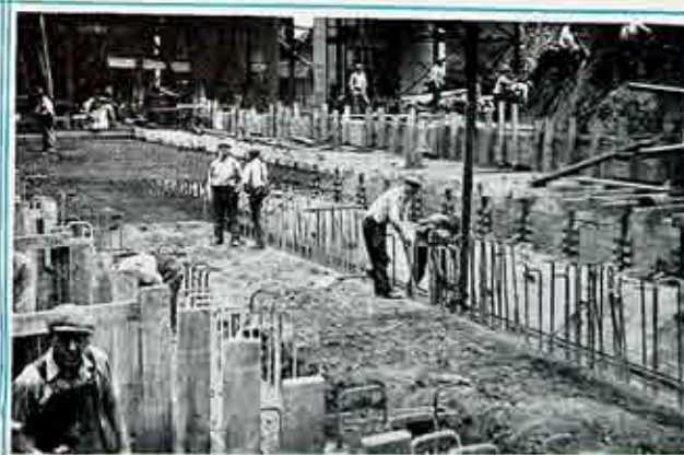
Scenes at West Station Gas Manufacturing Plant. Top, where the 37 new Koppers Becker type ovens, the third battery, hooked on to the CO ovens of the same type already in service; center, the new tar distillation process at the end of the second battery of Koppers ovens, and bottom, constructing the foundations for the new ovens, all these activities being supervised by employees from the Engineering and Gas Manufacturing departments alike.
