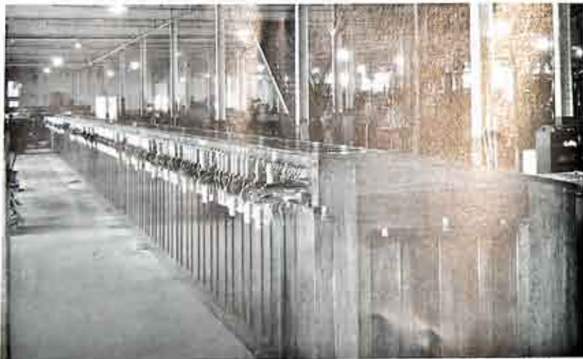
A G-R-S Electric Interlocker, the largest machine of its kind ever built. This interlocker was recently installed in the new Central Terminal at Buffalo, New York.
