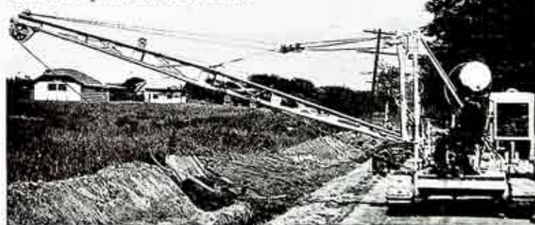
The use of modern equipment for digging and filling in trenches was an aiding factor in the Company's installation of over 284,000 feet of new gas mains last year.
