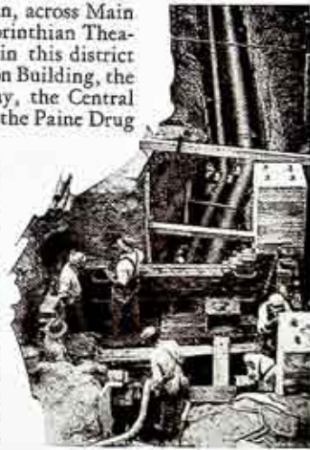
Steam manhole in line serving the General Railway Signal and Symington Companies in process of construction. It is located just across the N. Y. C. tracks, at the south end of Station Nine's steam bridge.
