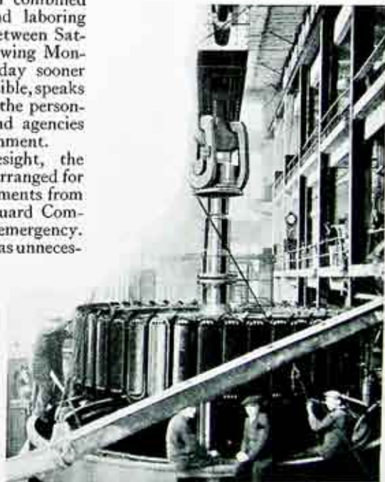
Figure 6. Installing rotor of new 22,500 H. P. generator at Station 5. Note huge equalizing bar at top of illustration. This bar makes possible the operation, in synchronism, of both cranes at Station 5, with a total lifting power of 135 tons.
