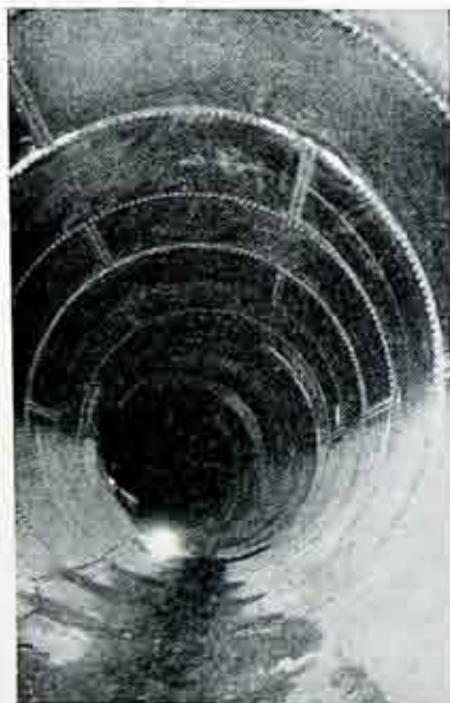
Figure 5. Newly constructed section of No. 3 penstock leading to 22,500 H. P. generator. Butterfly valve in distant shadow.
