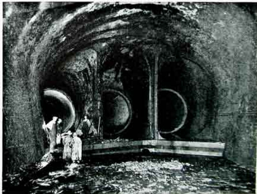
Figure 2. Extreme northern end of tunnel; at the extreme left, upstream end of No. 3 penstock from which the bulkhead was burned away to permit tunnel water to pass through newly constructed tunnel section, through butterfly valve to the new 22,500 H. P. generator recently installed at Station 5.
