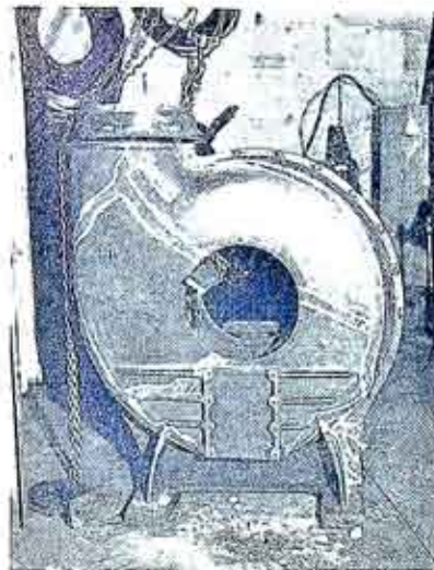
The blower set in position, ready for welding. The chalk marks indicate the breaks.
