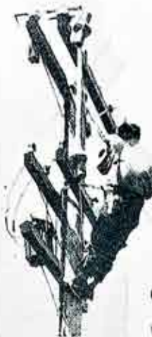
These three men, Messrs. Roy Maken on the pole, Edmund Tompkinson and Bernard Cahill, are installing an anchor guy in accordance with specifications shown in the diagram on the opposite page.
