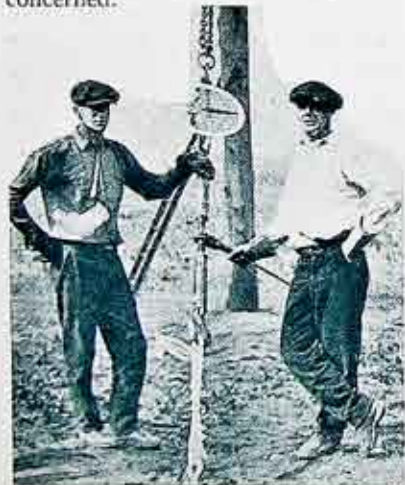
Testing a small concrete anchor block and a six-foot rod. 9,000 pounds was sustained in sand with only a two inch outward creepage. Fourteen similar tests were made of various type anchors placed around the pole shown above. Employees shown here are Messrs. Leon Atkinson and Charles Bruman.
