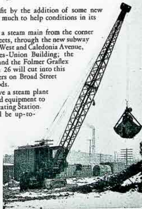
One of the Company's large locomotive cranes breaking ground for Station 9 Steam Plant, Lincoln Park.
