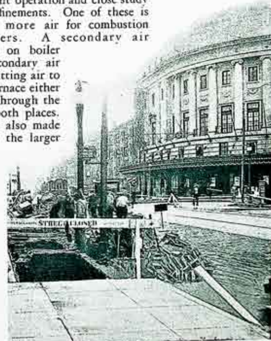
Widening Main Street East and other city streets made necessary the alteration of gas and electric underground installations, manholes and lighting poles.
