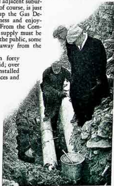
Much of the Winton Road gas main subway installation extends through solid rock, which complicated the work.
