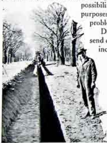
Trench Dug by the Company's Large Trenching Machines Utilized Mostly in Rural or Suburban Digging.
