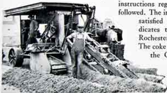
Fig. 1: Small Trenching Machine which cuts down the Cost of Digging Trenches for Gas Main and Electric Duct Installations.
