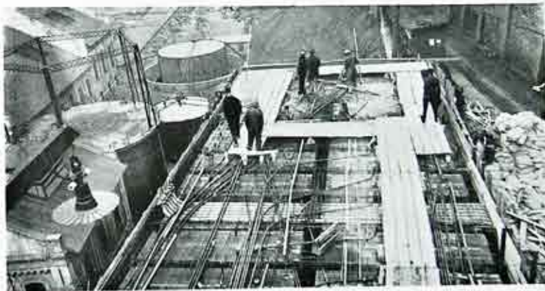
A Glimpse of the Addition to Station 34 Which Is Nearing Completion. A Section of East Station May Be Seen in the Left Background.
