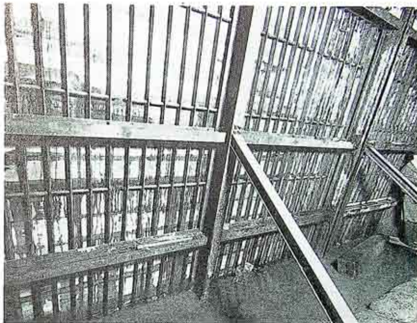
Fig. 2: Interesting Rack Construction. Note the Wide Spacing of Bars and Diagonal Bracing.
