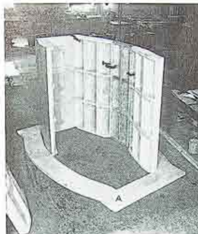
Figure 4, Showing Wooden Manhole Form in Construction. A, shows the Template Used in Marking out the Size of Manhole to be constructed.
