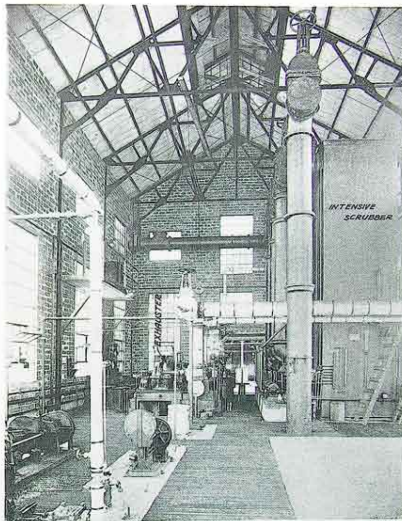
Fig. 1—Illustration of Exhauster and Intensive Scrubber at West Station Gas Works.
