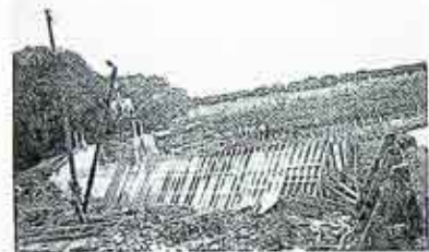
Fig. 2. New dam at Littleville under process of construction. The portion shown is the same as in figure 1. The spillway section is at the right but cannot be seen.
