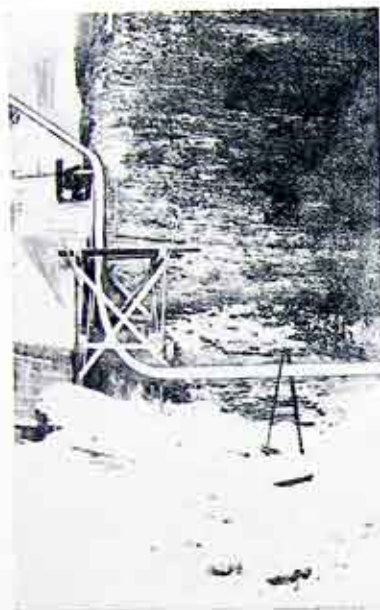
Fig. 4. Overhead portion of steam main running over penstock near Station 2A
