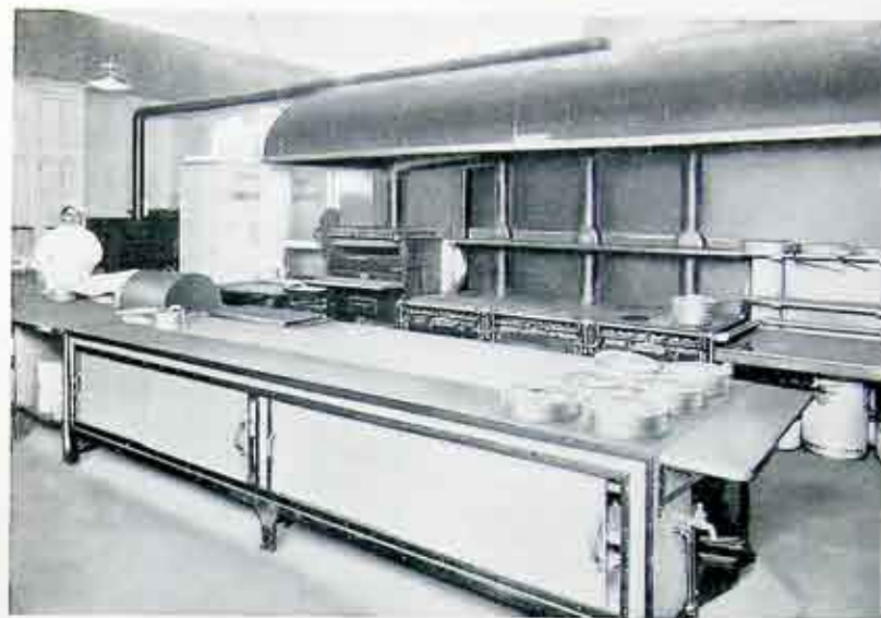
The above up-to-date complete gas kitchen equipment was installed at the Rochester Club on October 18th. The equipment consists of three sections of Garland Hotel Ranges, 1 Rex Ray Surface Combustion Broiler, 1 Vulcan Bake Oven, 1 40-gallon Stock Kettle, 1 Vegetable Steamer, 1 Battery of Coffee Urns with urn stand and cup warmer below, 2 Plate Warmers, 1 stove used by Pastry Cook, together with gas burner apparatus under dish washing machine. The gas consumed for the past two months totaled 484,000 cu. ft., costing about $160.00 a month. The club management and chef are very much pleased with the superiority of the gas equipment over the use of coal.
