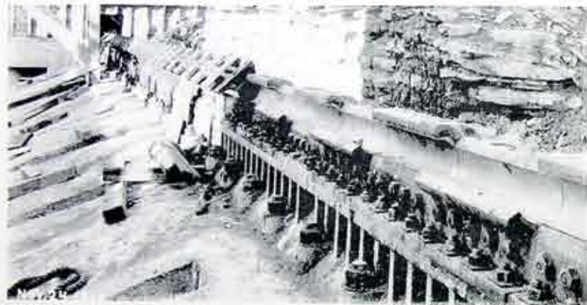
Fig. 3. Picture showing the construction of the large hinge required for one of the gates. Type "A" bearing projects on top, while type "B" bearing projects at the bottom.
