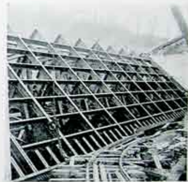
Fig. 5. Framework of sector gate showing deck prior to being covered with steel plate.
