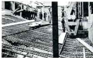
Fig. 4. Placing reinforcing steel in the concrete chamber into which the gate descends. Note the size of the drain chute.
