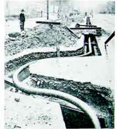
Fig. 2. View of Company's new steam main which runs from the Rochester Candy Works north on State Street to Jay, and thence west to the Shinola Company's Building. Note the U-bends used to take care of the expansion and contraction of the pipe.
