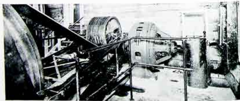
Fig. 1. 150 horsepower motor belted to a 75 ton refrigerating machine at the Kondolf Ice Company's plant. The operation is very smooth and efficient.
