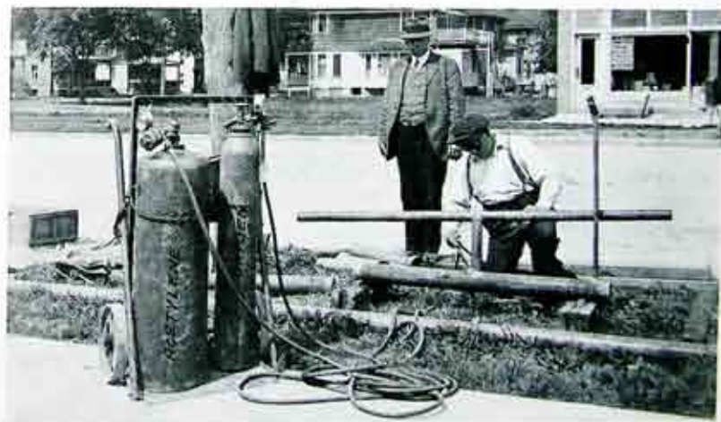
Fig. 3. Welding drip which was installed on East Rochester gas mains
