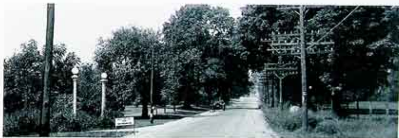
Fig. 1. Trench at side of East Ave. road on way to East Rochester. Sign reads "This pipe will carry gas to East Rochester"
