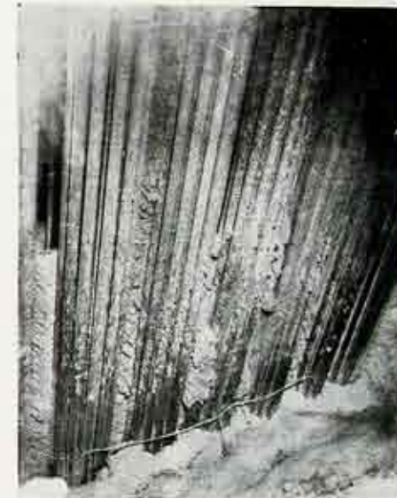
Front View of Tubes. Note Melted Ash Adhering to Tubes
