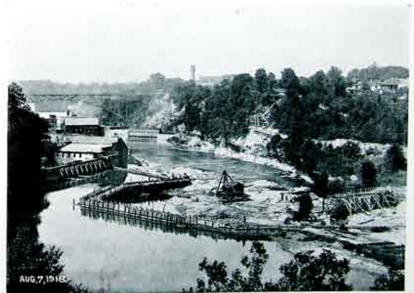
Fig. 3. Coffier dam at Station 15, where intake house will be located. Tunnel will start here and run about 1500 feet north to outlet at Station 5, shown in Fig. 2.
