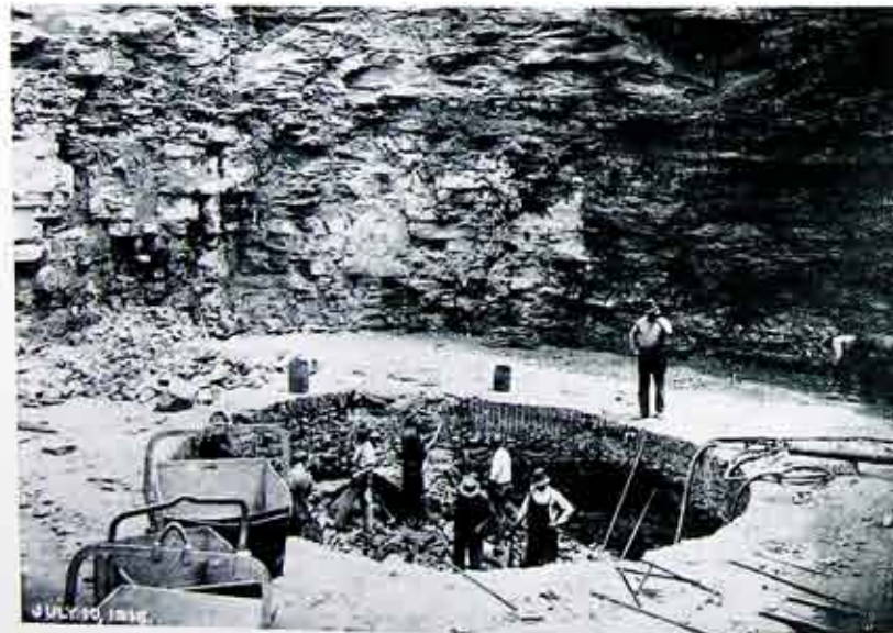
Fig. 1. Starting excavation for riser to surge tank. Shaft about 22 feet in diameter, and 100 feet deep to tunnel below.
