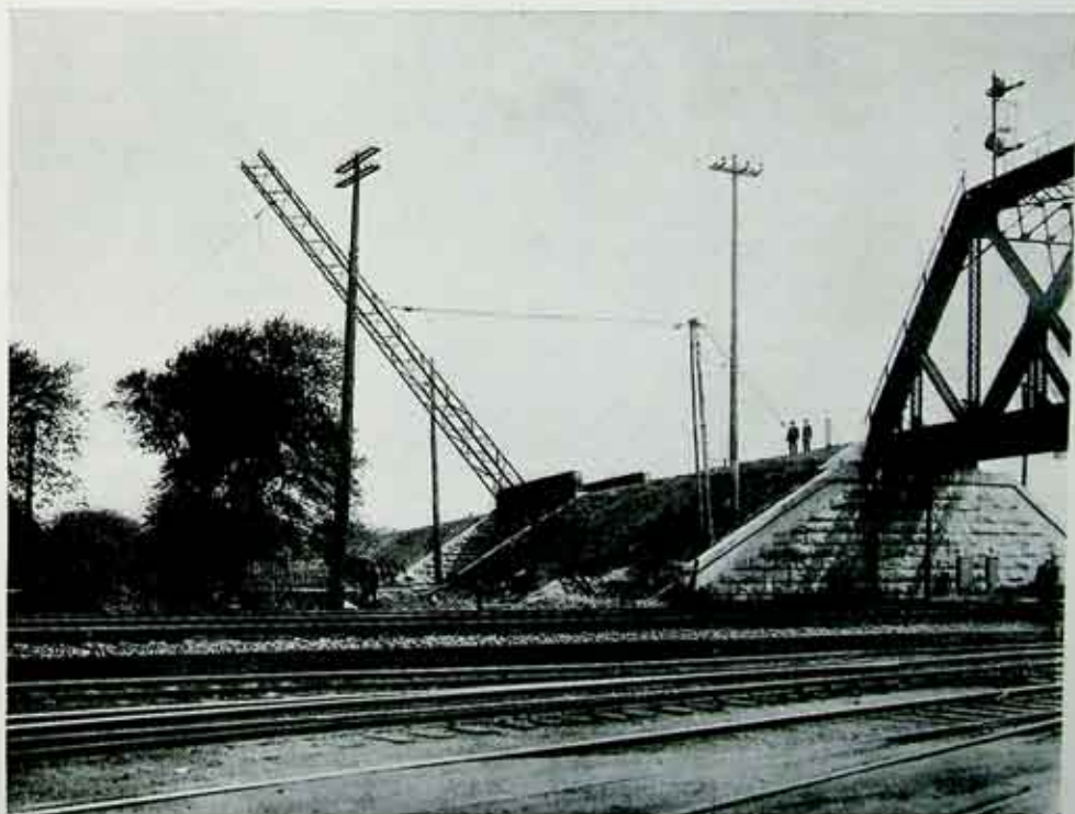
Erection of Transmission Line Tower at Crossing of 11,000 Volt Symington—Charlotte Line over Buffalo, Rochester and Pittsburgh Railway.
